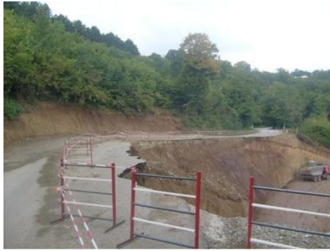
Fig 1. Road destroyed by Bodbe landslide
